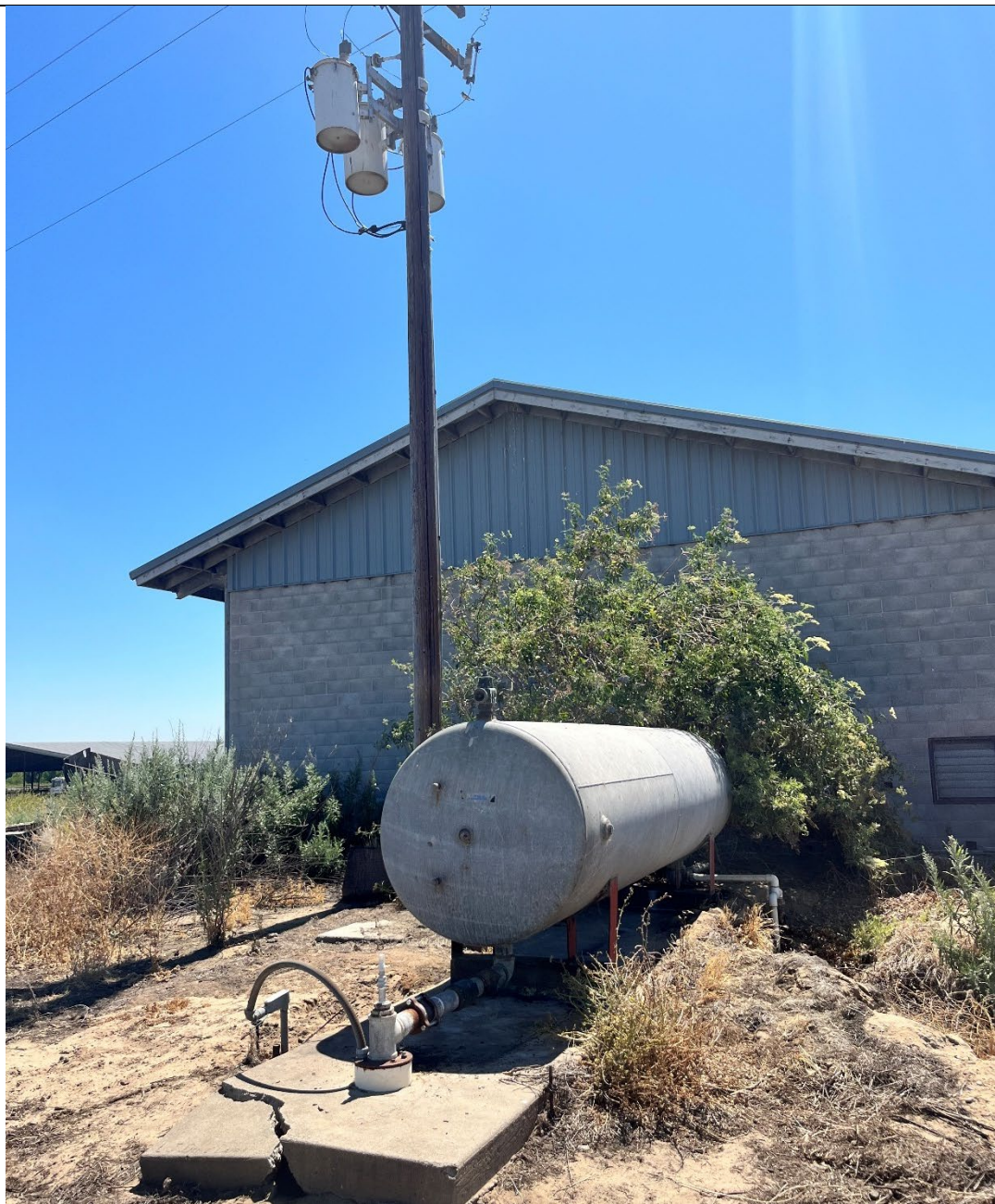
Water Well – to Preserve and Protect with power drop. No damage or disruption to this water service.
