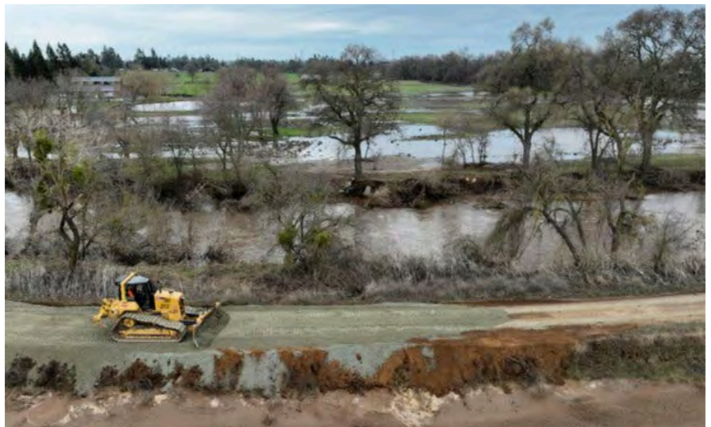
(Above) Repairs to a levee on the Cosumnes River near Wilton, Calif., that was breached by heavy rains on Monday. Fred Greaves/Reuters
