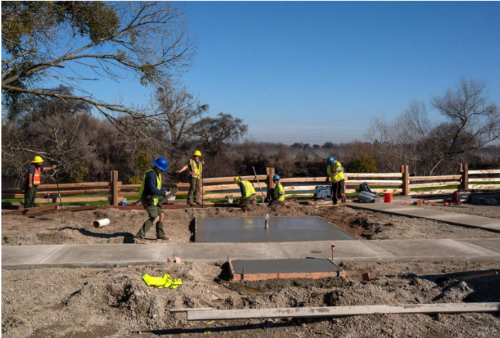
Workers build facilities for a new state park at Dos Rios Ranch Preserve near Modesto. (Loren Elliott / For The Times)
