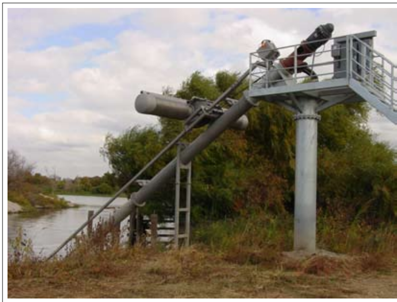
A high tech irrigation pump and fish screen enables River Partners to flood irrigate its new plantings, while protecting migrating salmon and steelhead in the San Joaquin River. Photo by River Partners.
